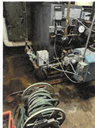
RIP steam boiler
