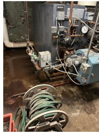
RIP steam boiler
