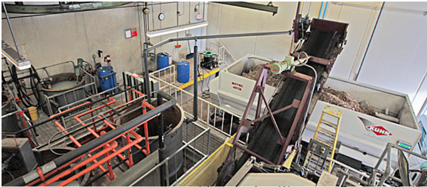
Ishpeming Area Wastewater Treatment Facility
