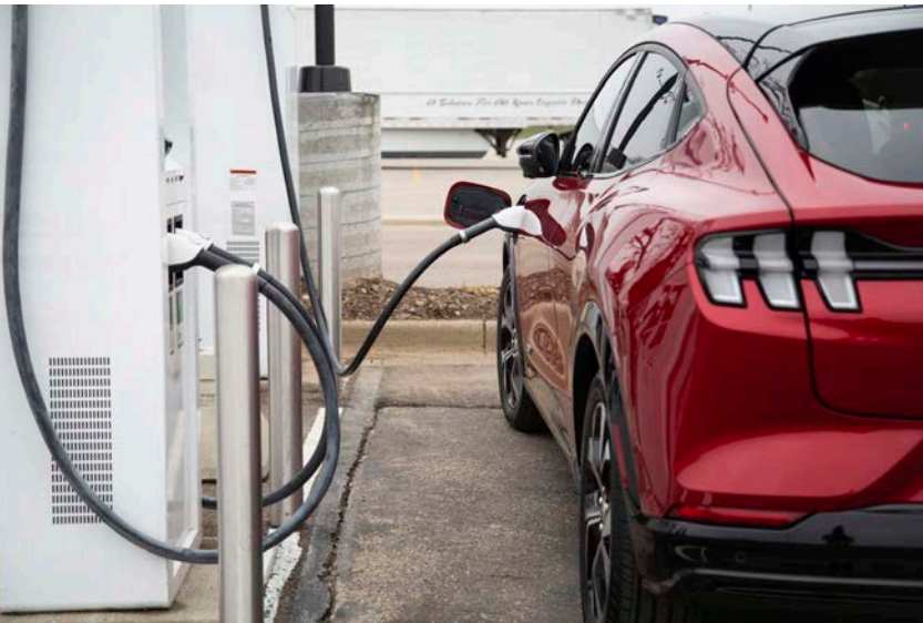
An EV Charging Station
