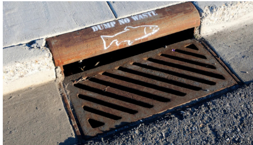
"Dump no waste" storm grate
