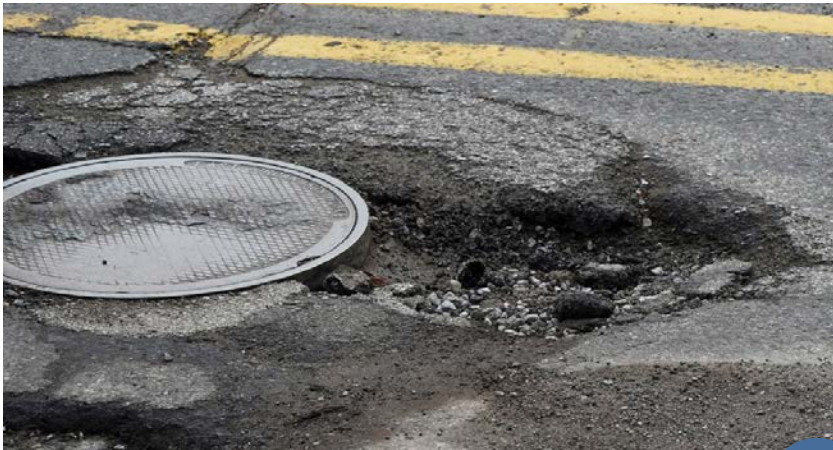
Pothole in Ishpeming
